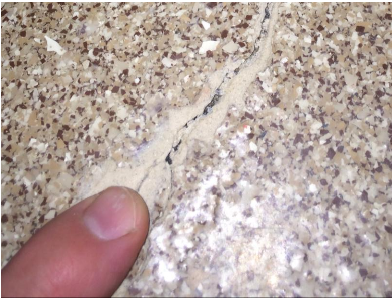
Figure 6 . Concrete has cracked after the application of flooring material.
