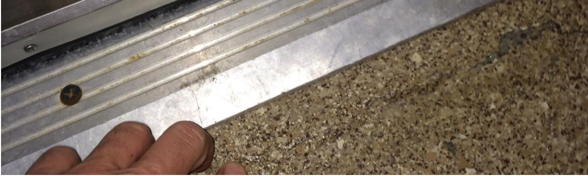
Figure 3. The interface between a footing and the concrete slab should be honored. In this picture the flooring contractor treated the slab and the footing as though they were monolithic, despite the fact they were not. This mistake is the flooring contractor's responsibility, as he should have anticipated the movement and addressed the detail with the owner.
